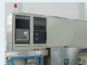
3S线用电控及瑞士仲巴赫在线控制系统 Electric control and In-line control (Zumbach) for Line 3S
